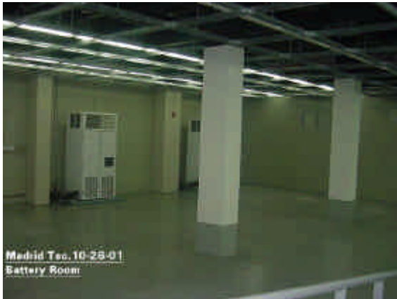
Madrid TEC – Battery Room
